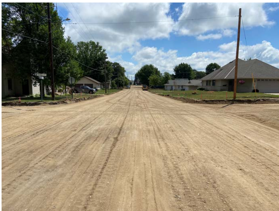
Left: Midland Avenue, looking east from 3rd Street. Roadbed is prepared for curb and gutter and driveway apron pouring.
